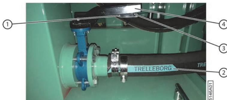
Fig. 55: The hydraulic valve
