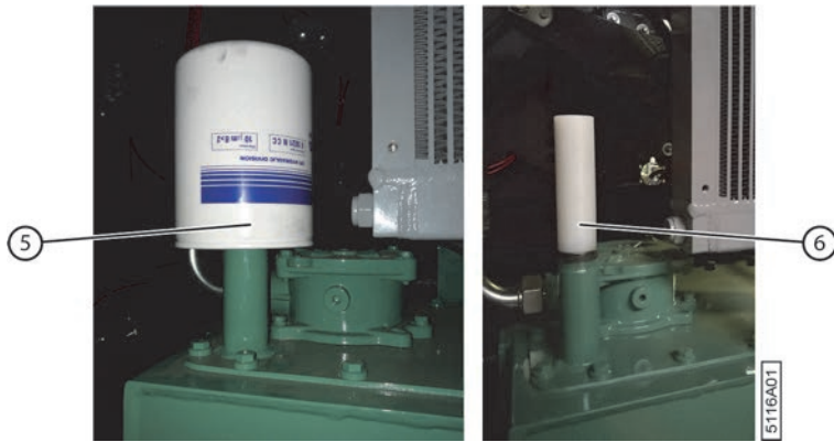
Fig. 16: The de-aerator and the anti-overflow device
